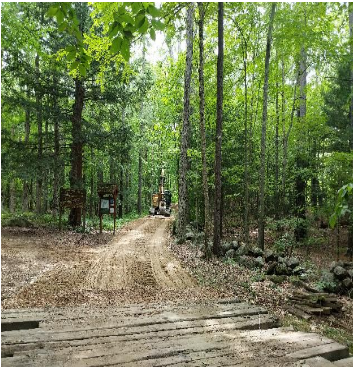
Fig 15: Crew actively installing access road off of Foss Farm road. Viewing northeast. (8-06-19).
