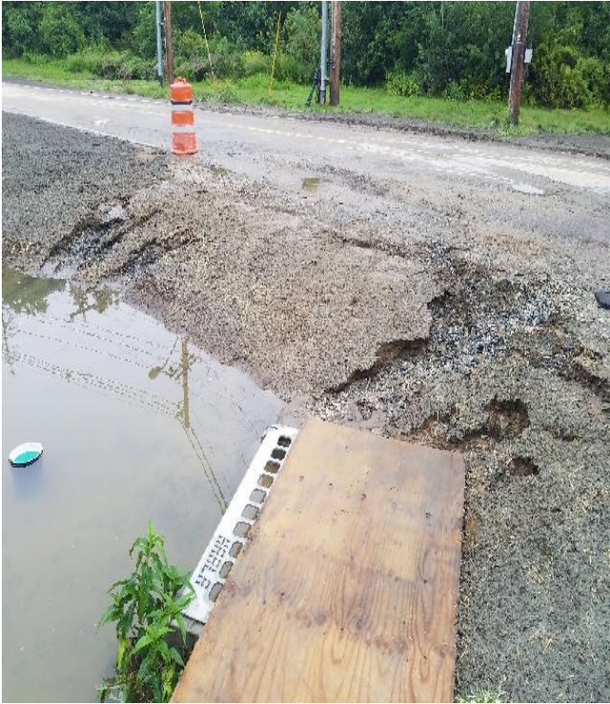
Fig 25: Slope erosion at the rain garden. Viewing northeast. (8-08-19).
