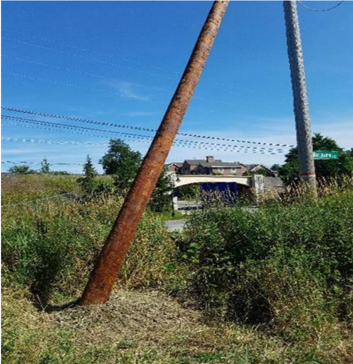
Fig 13: 380 line push brace temporarily installed in wetland DW67 with minimal wetland impacts. Viewing south. (8-05-19).
