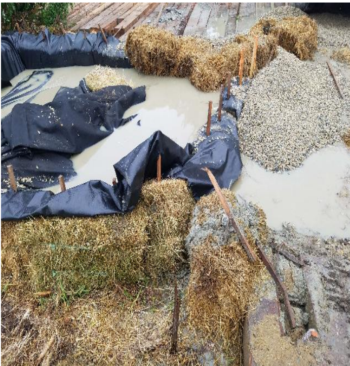
Fig 23: Newly installed dewatering apparatus for trenching activities through Gregg Hall Rd. Viewing east. (8-08-19).
