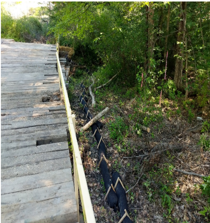
Fig 11: Filter sock installed on the east side work pad at Str. 28. Viewing north. (8-05-19).
