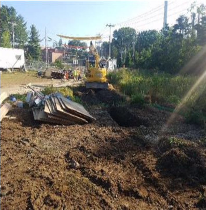
Fig 17: Beginning to trench across the road leading to Gregg Hall. Viewing north. (8-06-19).
