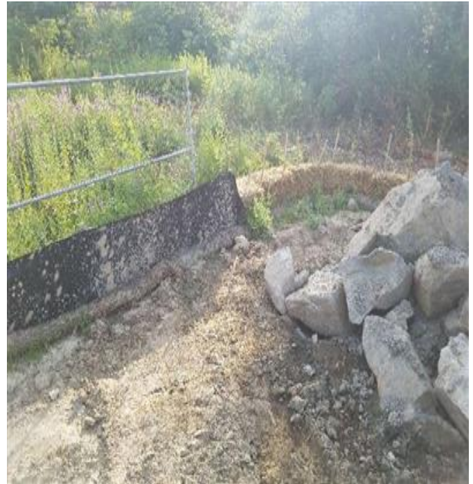
Fig 8: Straw bales installed in the wrong location in the Waterworks Rd laydown yard. Viewing east. (8-03-19).
