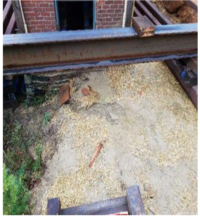
Fig 22: Slope erosion at cable house cont. Viewing west. (8-08-19).
