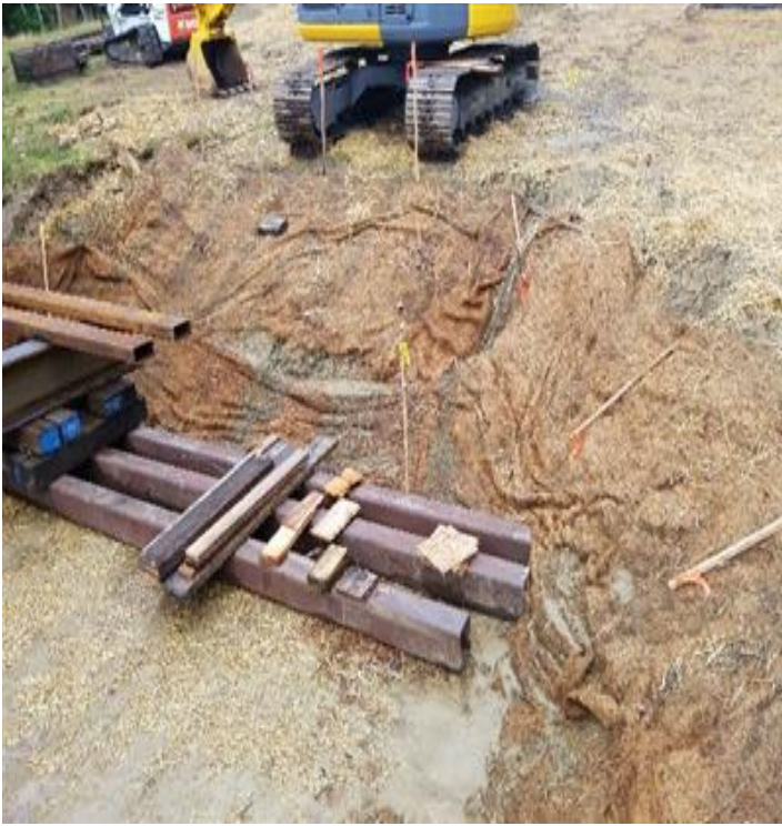
Fig 21: Slope erosion at cable house. Viewing west. (8-08-19)
