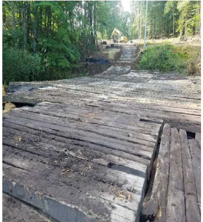
Fig 4: Work pad over wetland DW49 and slope adjacent to wetland DW49. Viewing south. (8-01-19).
